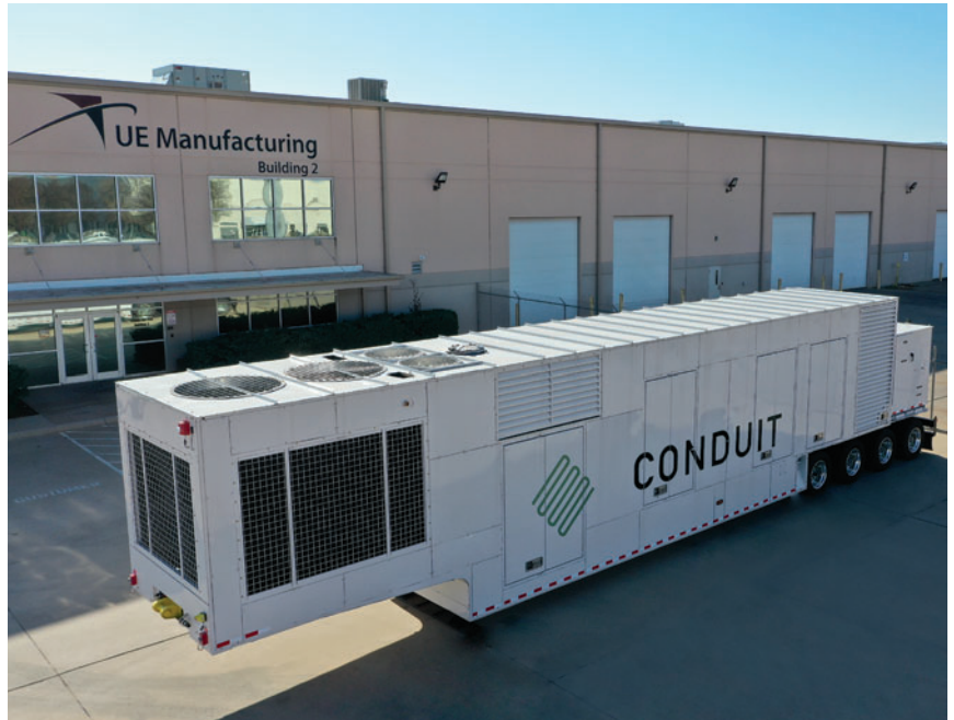
Mobile 2.5 MW natural gas powered generator for micro grid power applications
