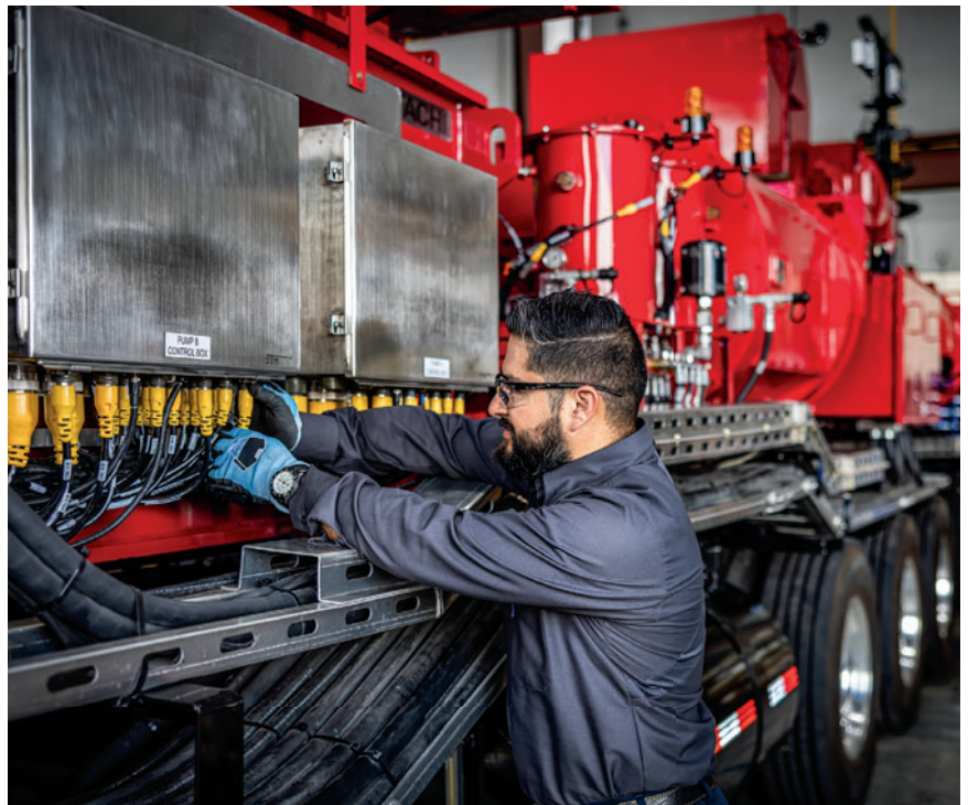
Stewart & Stevenson Generation 5 Electric Fracturing System.
